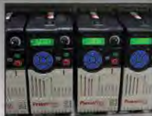
Priority One® consolidates and integrates all facets of the production line into one comprehensive control operating system.
